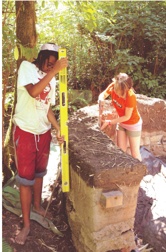
Xuny Haley and Amy Helmuth building a cob house at the 2007 Eco-Forestry work camp at Camp Myrtlewood in Oregon.
